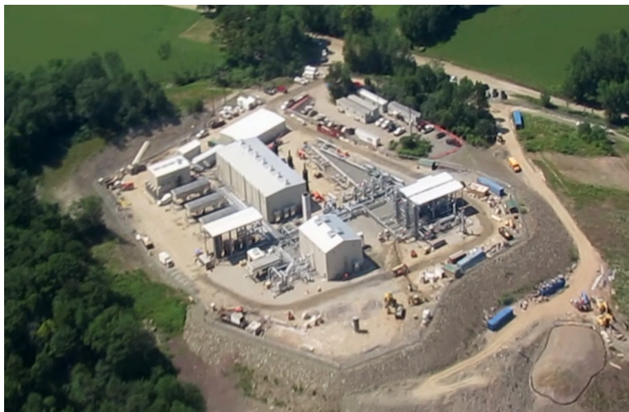
This is a photo of the similar 21,000 horsepower Williams Central Station in Susquehanna County under construction.
